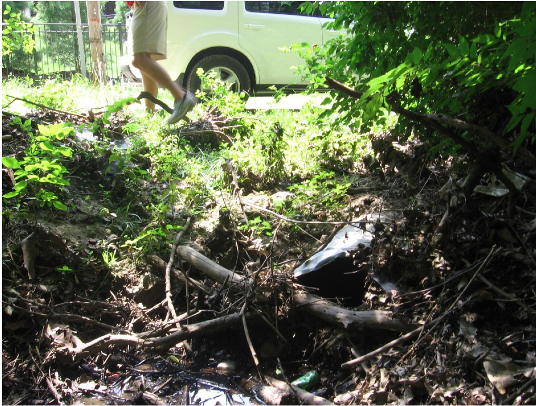
Looking west at the existing culvert crossing from the potential detention area east of Sellenriek Road
